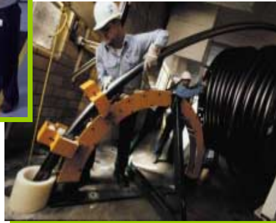
HTS Cable Project Development
