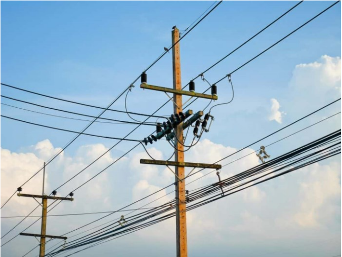
Typical distribution line (<50 kilovolts [kV])
