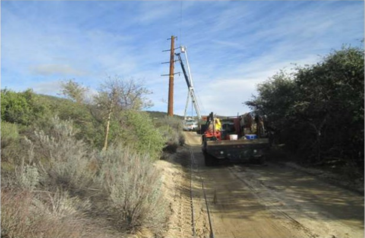
Typical power line (50-200 kilovolts)
