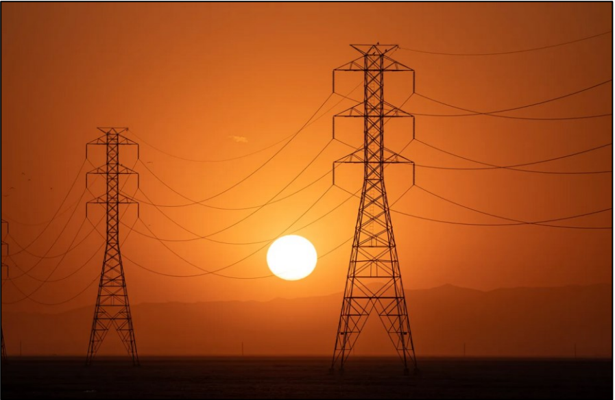
Typical transmission line (>200 kilovolts)
